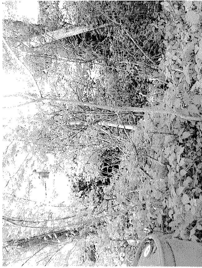
Description: Downstream channel for emergency spillway.
